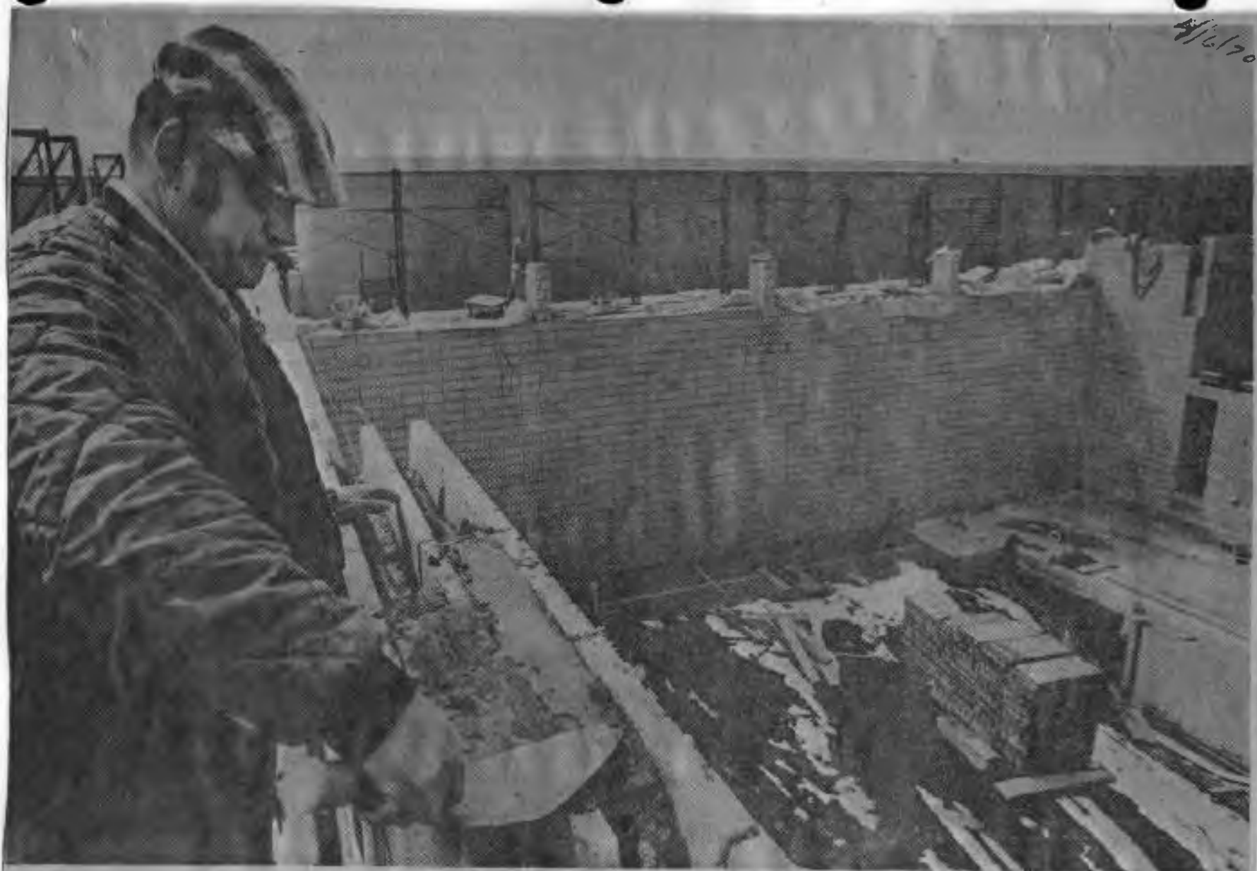
LEVELING OFF THE MORTAR , Jerry Dykyj of Chicago continues work on the new Wheeling Park District indoor pool being built adjacent to Wheeling High School on Hintz and Elmhurst roads. Work is ahead of schedule on the pool which is expected to be completed before school starts next fall. Fees for use of the indoor pool and the district's outdoor pool were established by the park district board Thursday.
